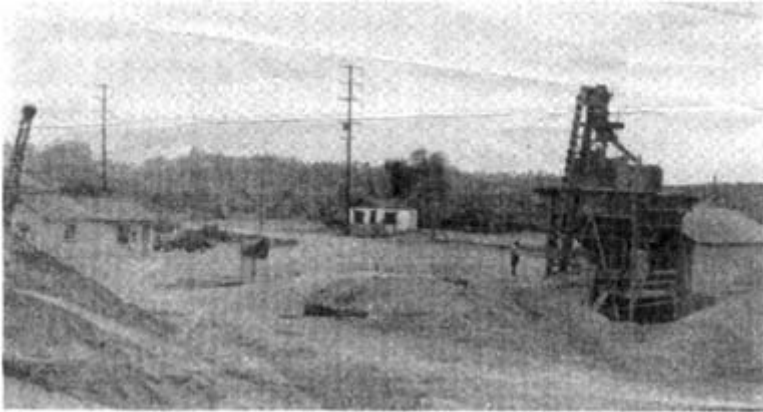
• The batching plant on the premises of the Holliday Rock Products Company at Colton, Calif.
